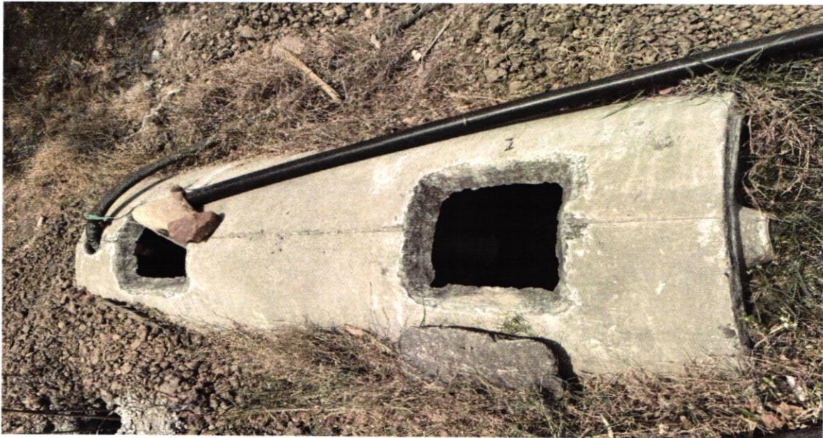
Figure 2.2 :- Water Storage Tank and capacity of College Campus
